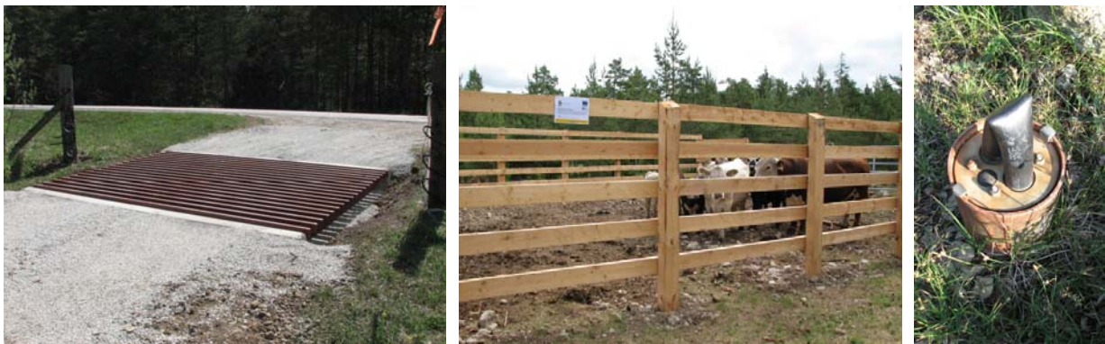
Pictures of constructions facilitating animal care that was performed within the LIFE-project: one of the cattle grids placed near the main road, one cattle pen, and one of the drilled waterholes.
