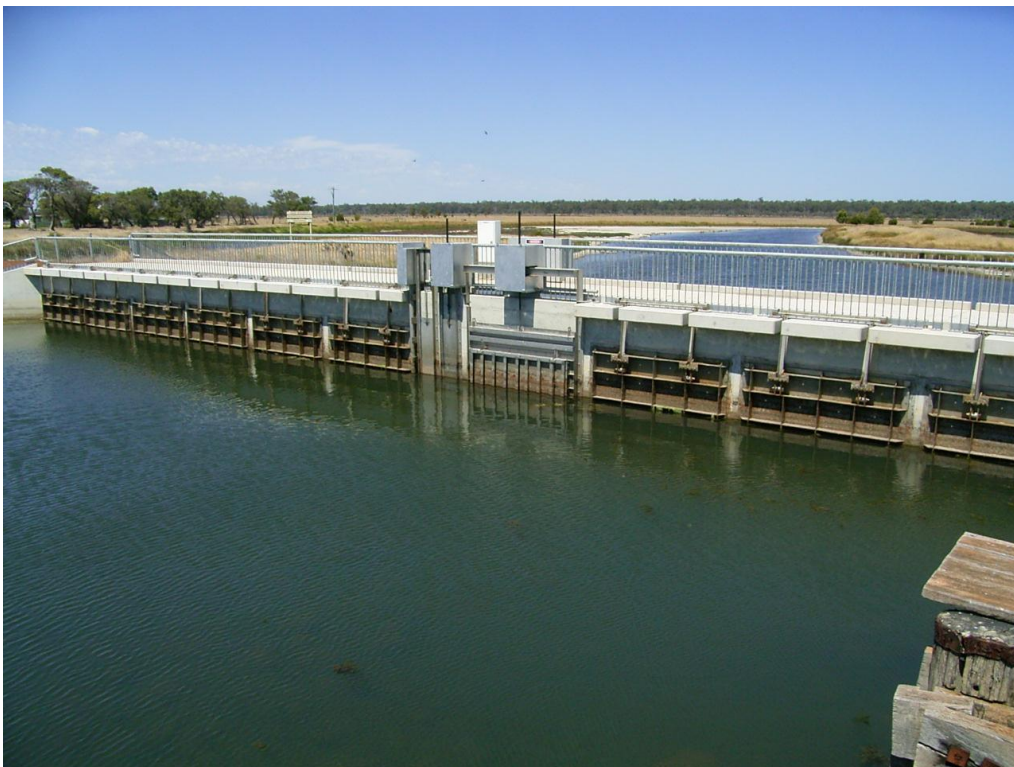
Floodgates on the Wonnerup Estuary, Jan. 2007 (Andrew Storey)
