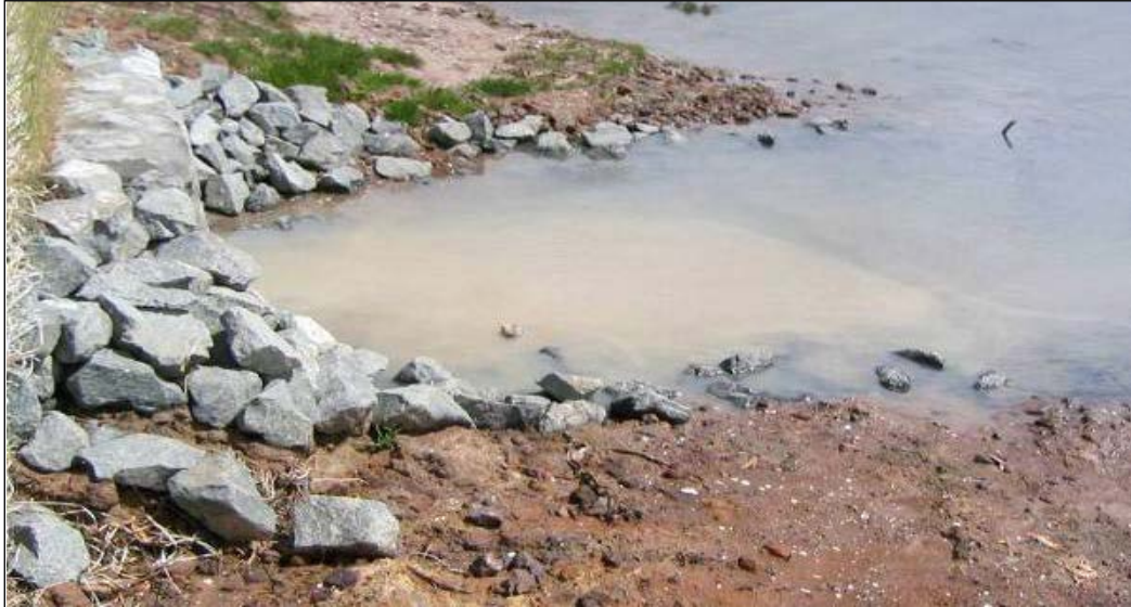
Figure 8 A stormwater drain discharging sediment directly into Orielton Lagoon
