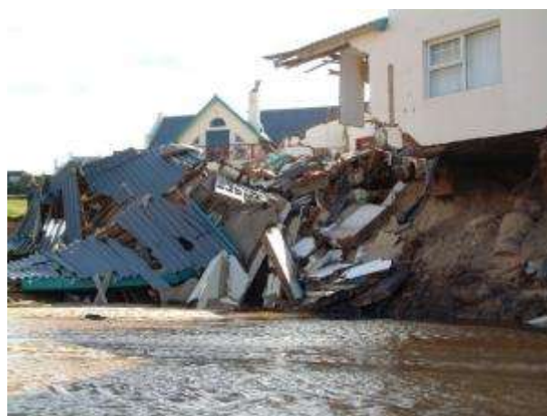
(c) Flood damage
