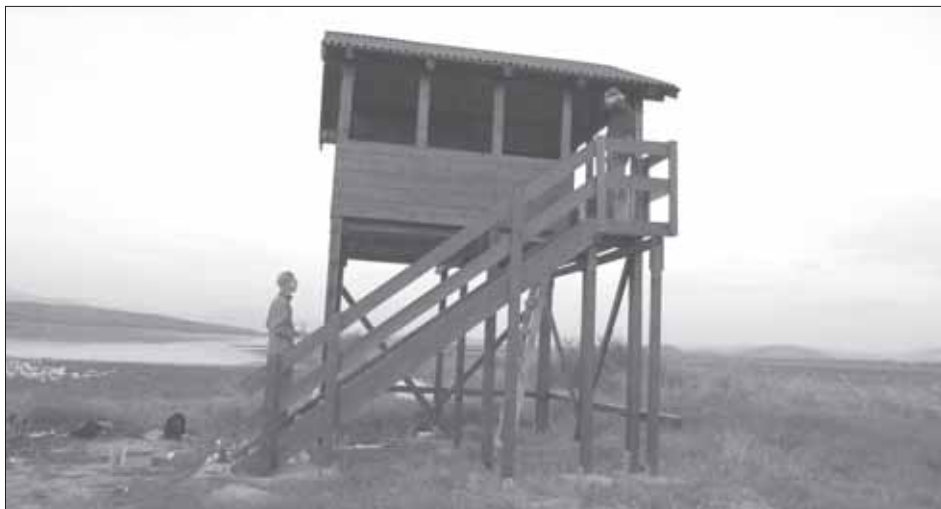
Fig. 24: Construction of the central observation tower along the inner visitor trail on the dike between Jezereo 1 and Jezero 2. 25 September 2006, Solana Ulcinj (Photo: M. Vernik).
