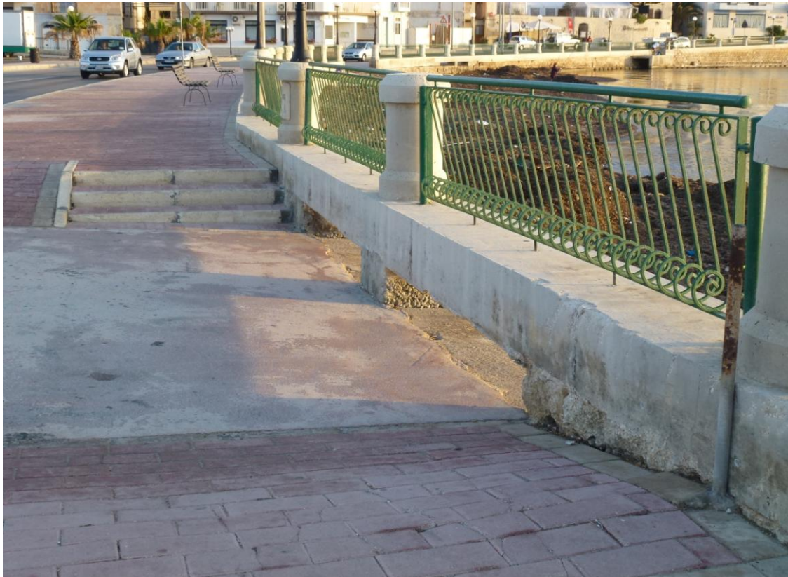
Figure 32: Discharge point at Xemxija Bay
